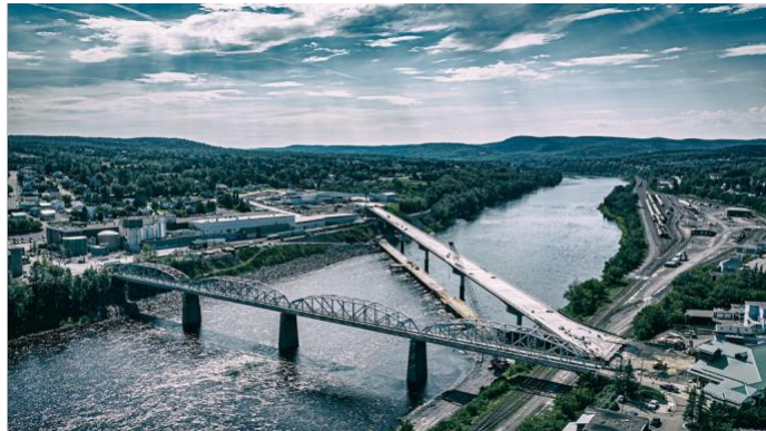
Madawaska International Bridge. International bridge spanning the St. John River between Madawaska, ME and Edmundston, NB. Opened in 1922, the original bridge is limping along to its end of 100 year useful life. The new bridge, under construction in the image, is due to open in 2025, rated as well at 100 year useful life. Along with the new bridge is a new US border crossing station, 1,400 feet upstream from the original station.
